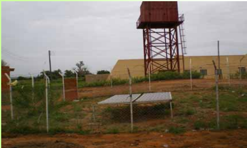
Solar Water Pumping for Students in Sokoto, Sokoto State
