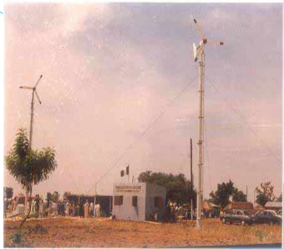
5kW aero generator in Sayya Gidan Gada, Sokoto State
