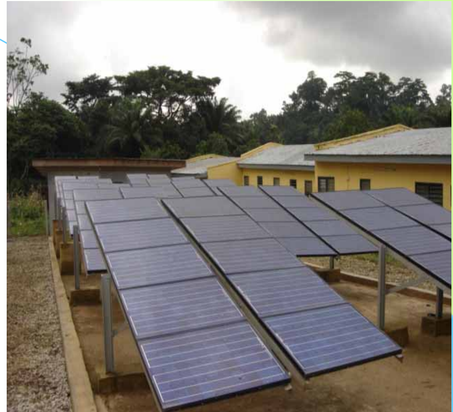
Solar PV at Ilaje, Ondo State of Nigeria
