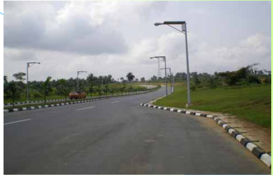
Solar Street Lighting in Uyo, Cross River State
