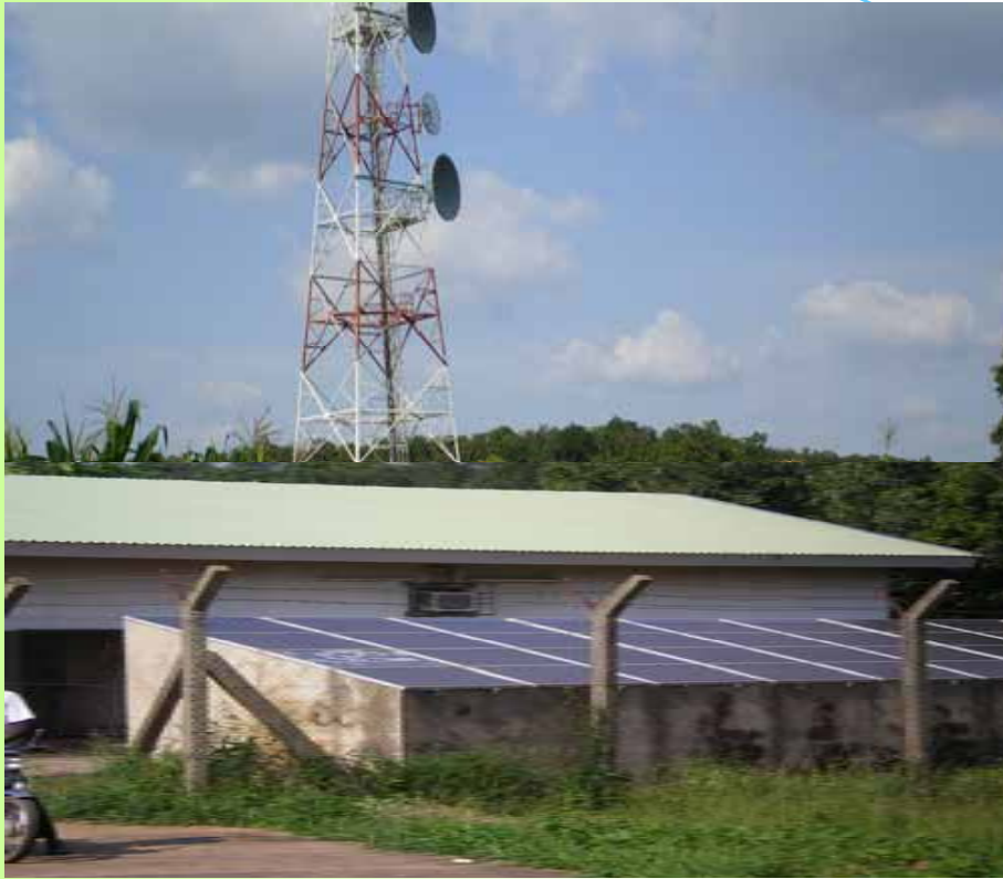
Solar PV for Telecommunication 20km Kaduna-Abuja Road
