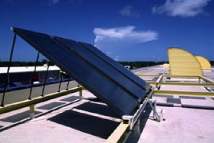
Businesses that use hot water can save money by installing solar collectors on the roof.
