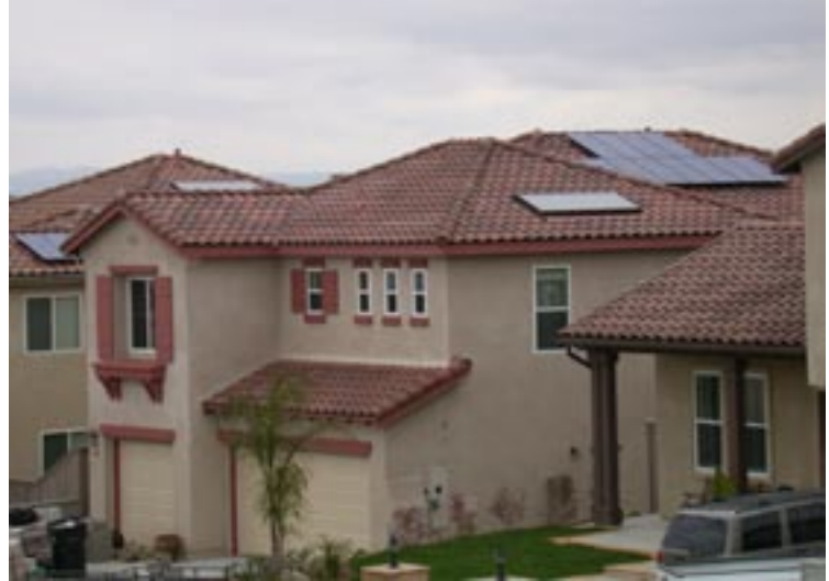
These San Diego homes are using the sun for both hot water and electricity. The solar hot water collectors are the single rectangles that look like skylights, while the larger array in the back is a photovoltaic system.
