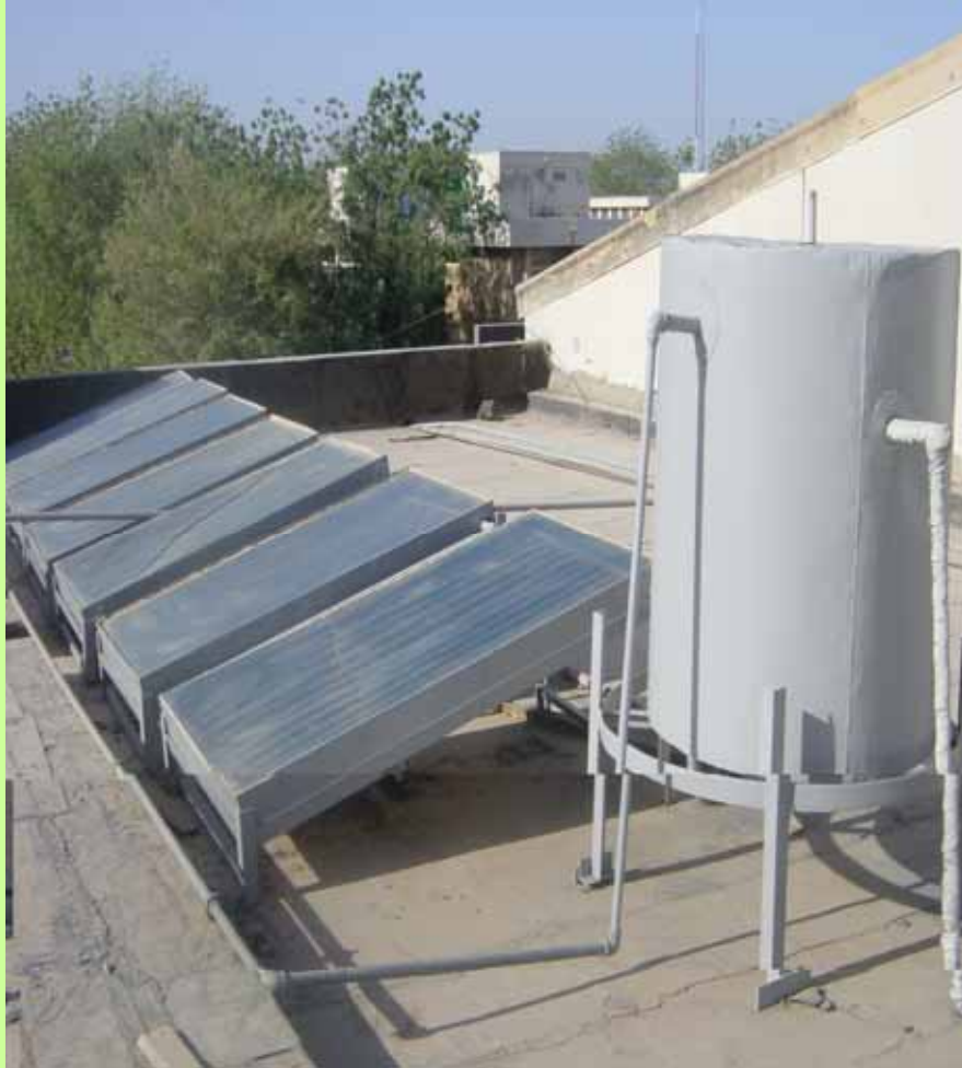
Pilot Water Heater at UDUTH by SERC, Sokoto
