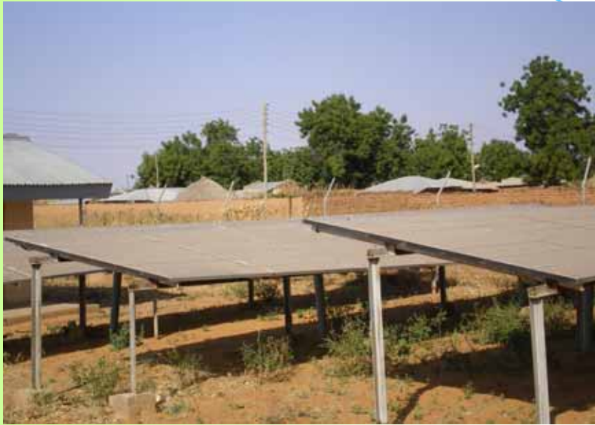
Solar PV mini-grid in a village in Sokoto, Sokoto State
